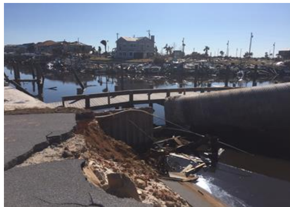
Figure 36. City canal opening showing extensive damage post Michael
