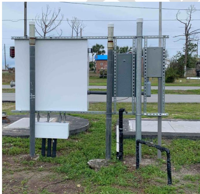
Figure 66. Wastewater Lift Station PS - 13
